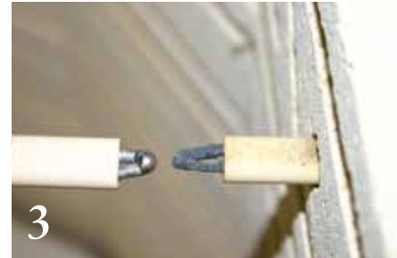
3 Check the thermocouple(s), for excessive oxidation.
